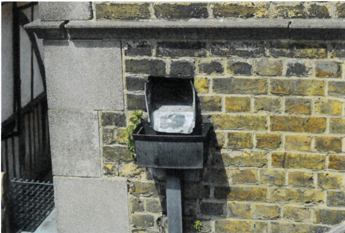
The lead chute could usefully be redressed.
