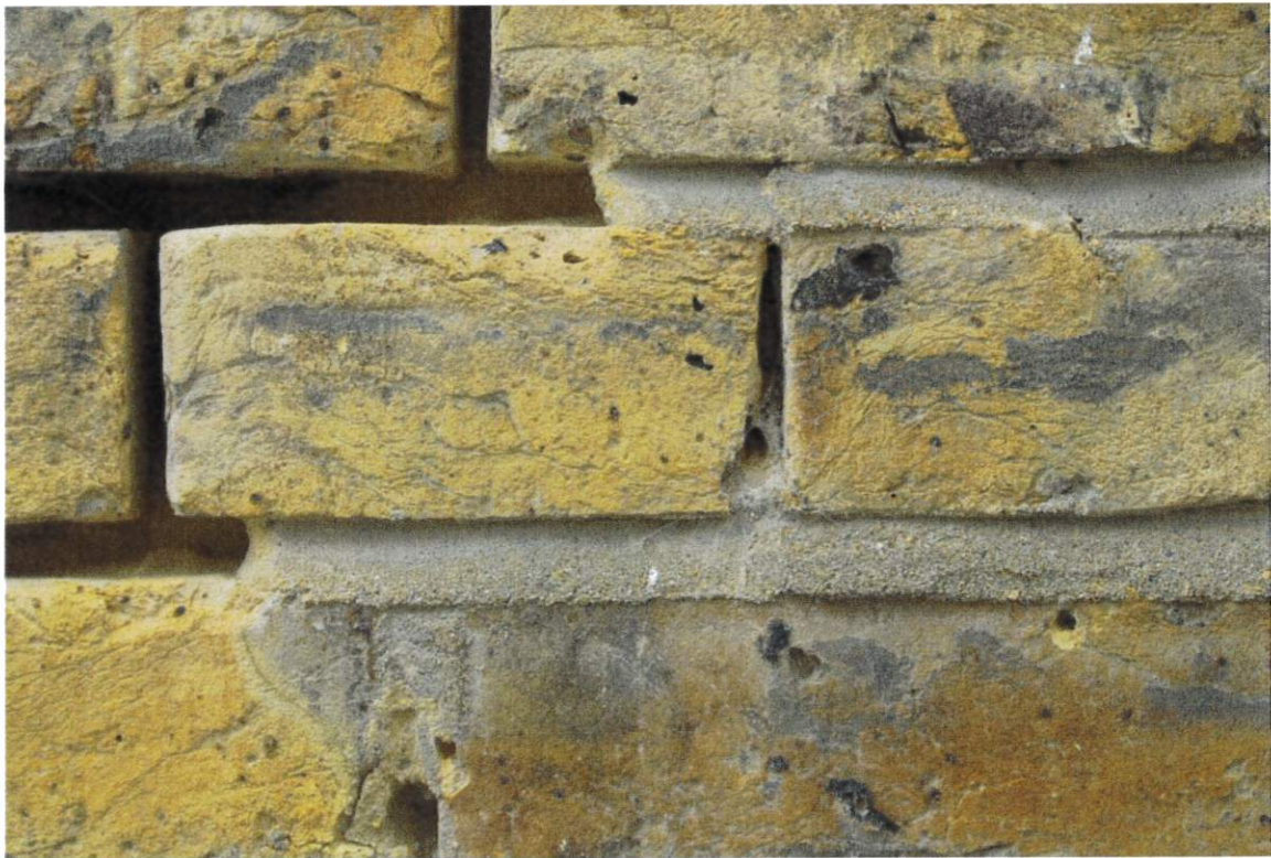
Erosion behind cement mortar pointing.
