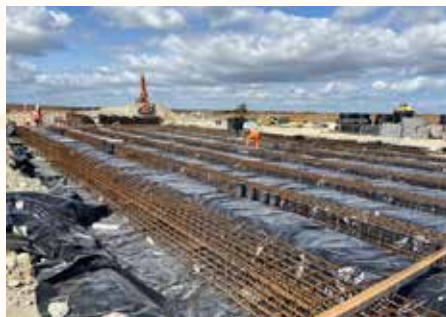
Electrical area within bund
