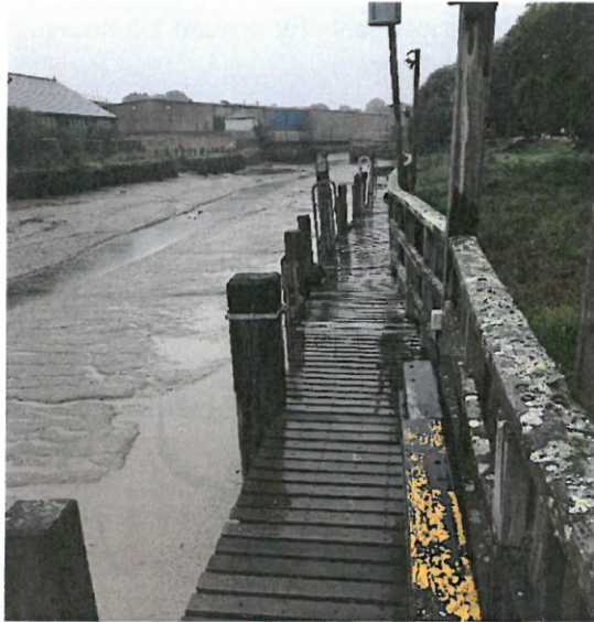
Photo 2: Failure of jetty structure
