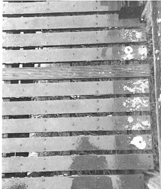
Photo 3: Deck board surface and organic growth
